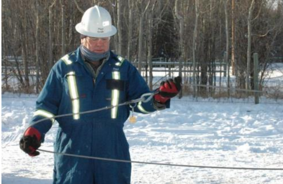
3.8.3. Keeping the cable separated grasp cable firmly & walk towards the desired anchor position.
